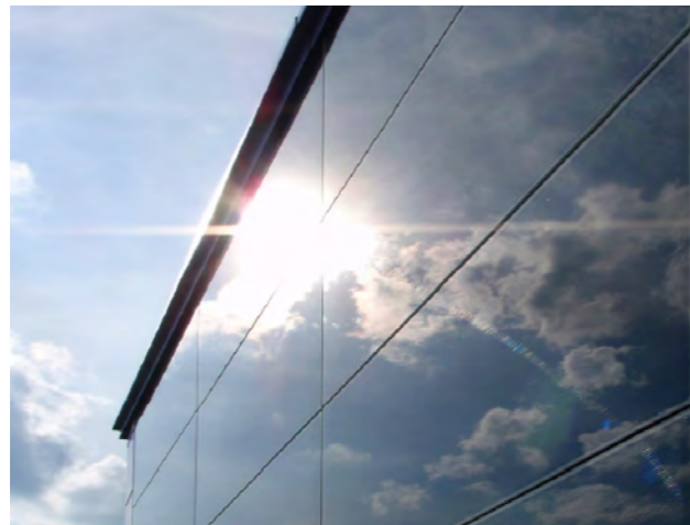
Fig.6 Building integrated solar-PV (Ruukki)
