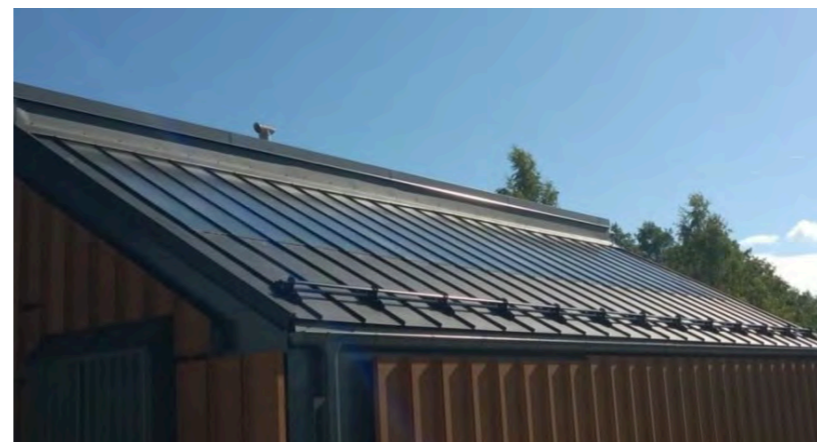
Fig.4 Roof-integrated solar heat collectors
