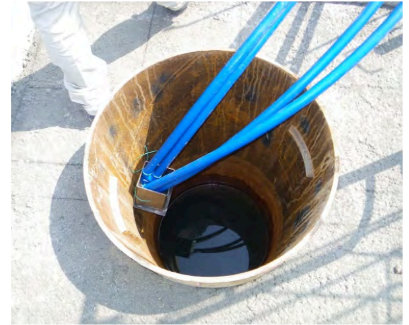
Fig.4 Insertion into U-tube pile started (with curing cover and weight at tip)
