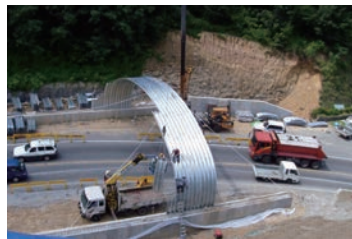
No traffic disturbance during installation
