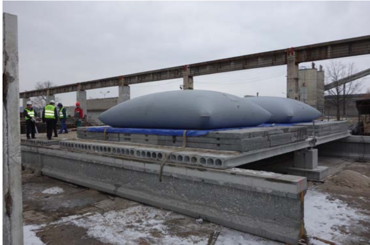
Fig. 5. Tanks filled with water on the road slabs aggravating the floor slabs and composite beam.
